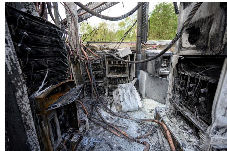
Damaged cabling and telecommunications equipment in Huddersfield, northern England, on April 17, 2020. The fire comes after a number of mobile phone masts have been set on fire amid claims of a link between 5G and the novel coronavirus COVID-19. | Photo by OLI SCARFF/AFP via Getty Images
