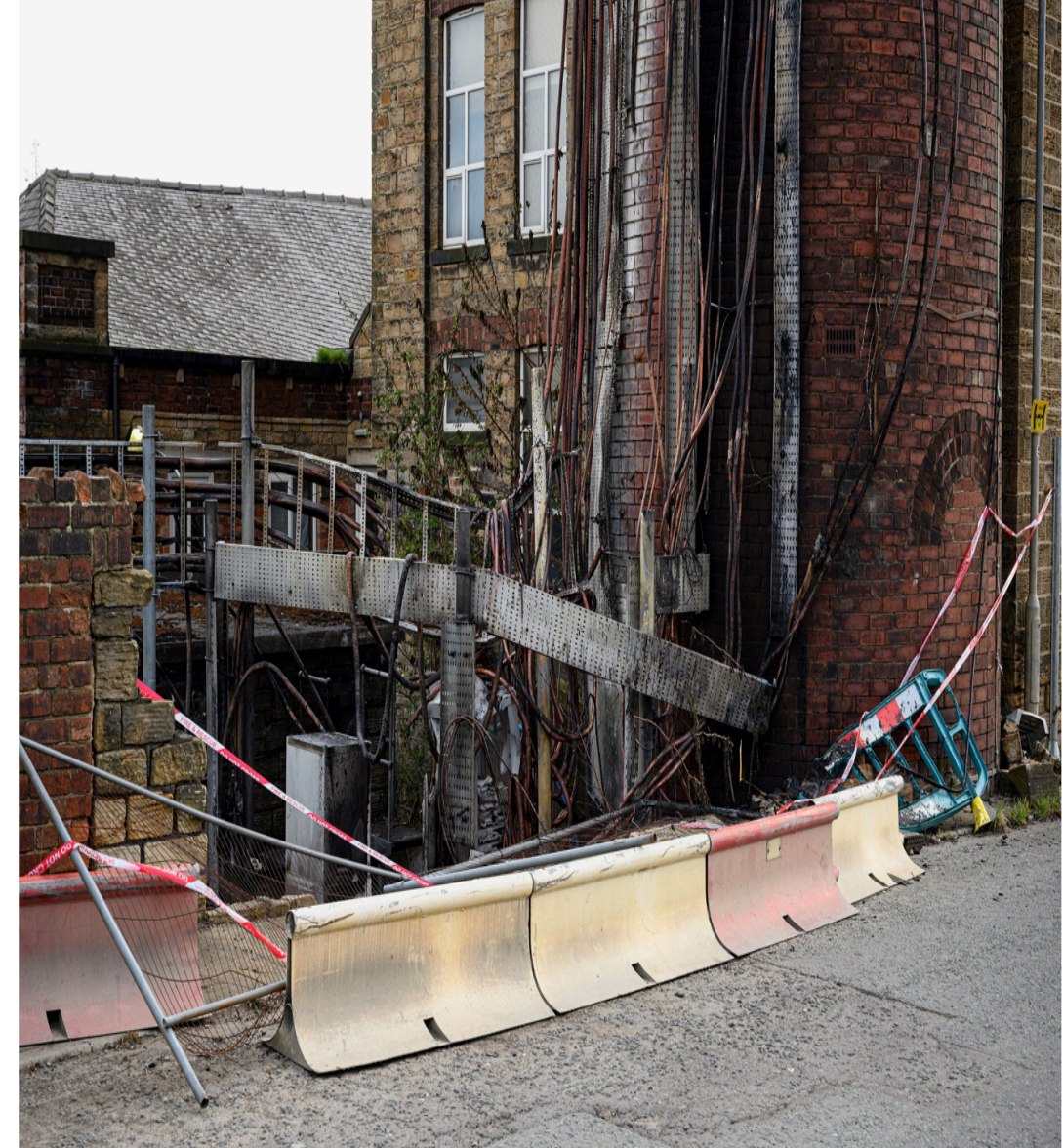
The cause of a fire that damaged telecommunications equipment in Huddersfield, England, is not yet known; several cell towers have been burned amid claims that 5G technology is related to COVID-19. Photograph by Oli Scarff / AFP / Getty
